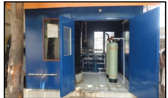
Interior of the RO plant
