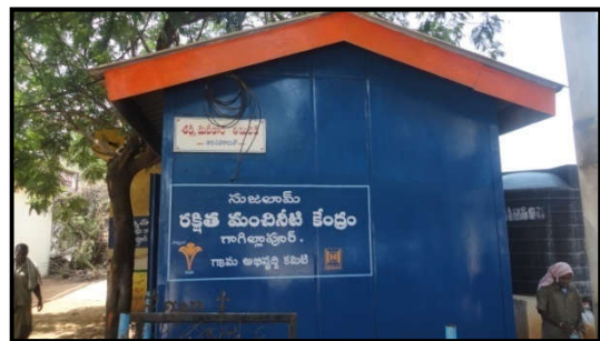
RO plant after revival in Main Village
